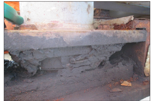
Existing bearing prior to removal shows excessive corrosion
